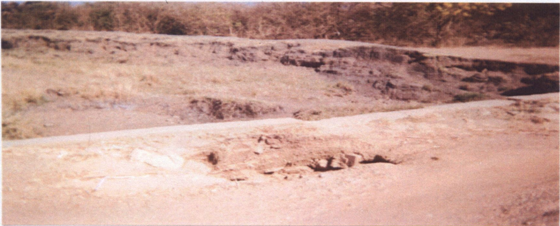
Plate 3: Lusowe bridge damaged at Mpanda village and river banks washed away by torrential rains that caused flooding in many areas of Zambia in 2007-2008 rainy season. (photo by the researcher)
