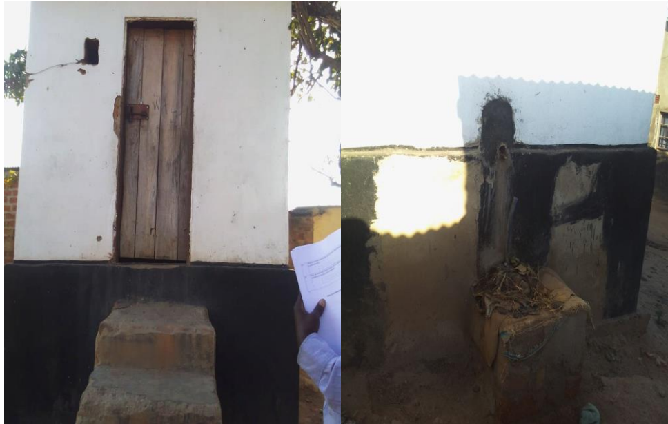
Figure 4.11: Improved type of toilets in the study area (LHS: Front view of the UDDT; RHS: Rear view of the UDDT). (Source: Field data, 2022)
