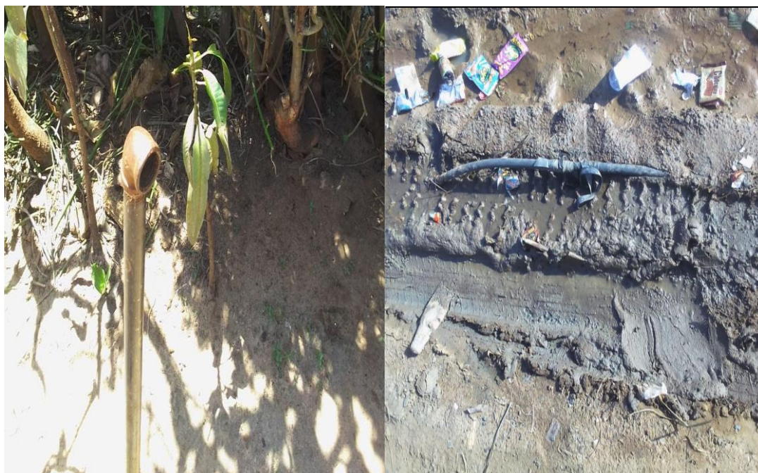
Figure 4.10: Vandalised facilities in the study area (LHS: A tap; RHS: Underground water pipe). (Source: Field data, 2022).
