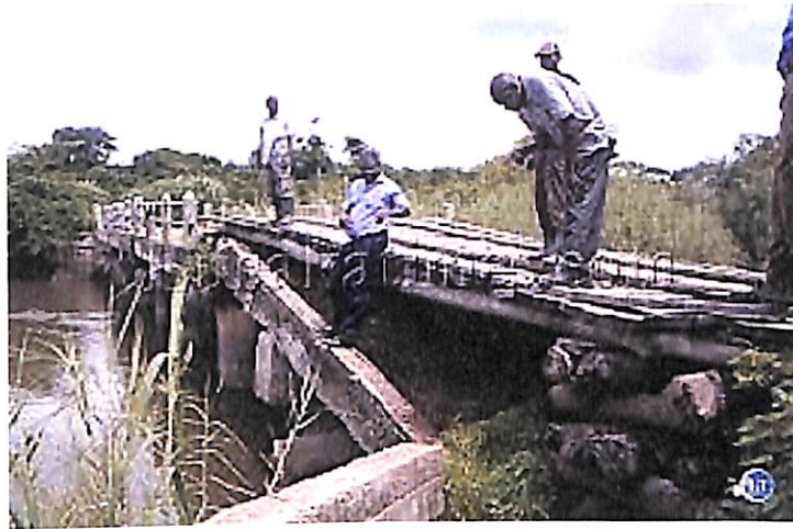
Fig. 156: Assessing damage to Kansangito Bridge, an important piece of infrastructure for this isolated area south of Kalumbila, Ntambu area, Credit: Lusaka Times, 21 st December 2012.
